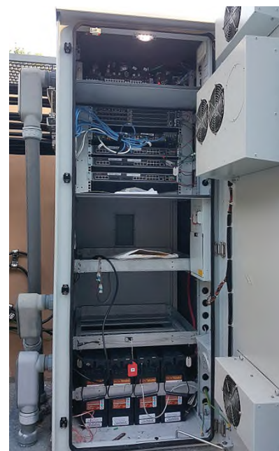
On-site OSP structure containing four Deka Fahrenheit HT170ET batteries.
