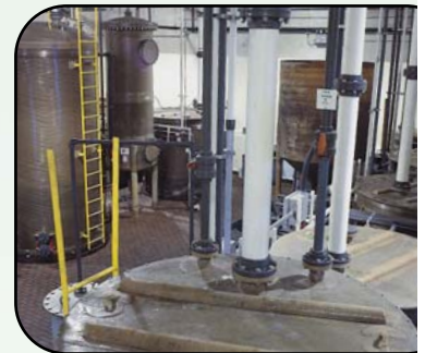
EPA-certified recycling facilities are utilized to protect you from risks.
